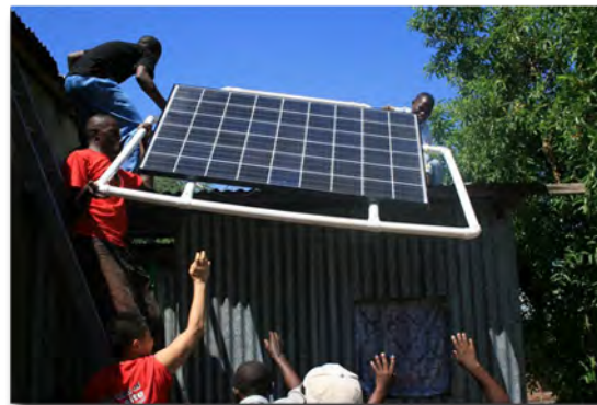
Solar panel placement
